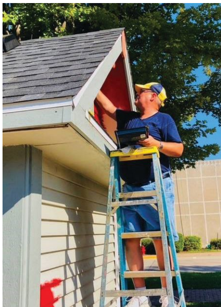
Morris Lion Steve Clark works on the rehab of Santa's House in Illinois.
