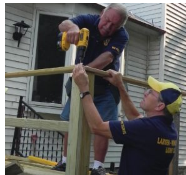
Lions Leon Harder and Kim Jansen secure a rail section for the 1,000th ramp.
